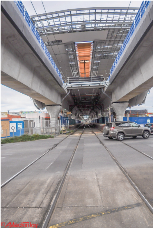
View looking along the existing tracks with Hughesdale Station overhead Photographs by Alan Mackinlay
