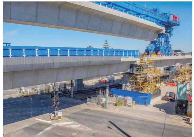
The last beam being lowered into place at Poath Road using the straddle carrier.
