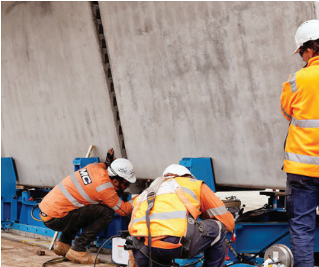
Assembling a beam of match cast segments to form a bridge beam.
