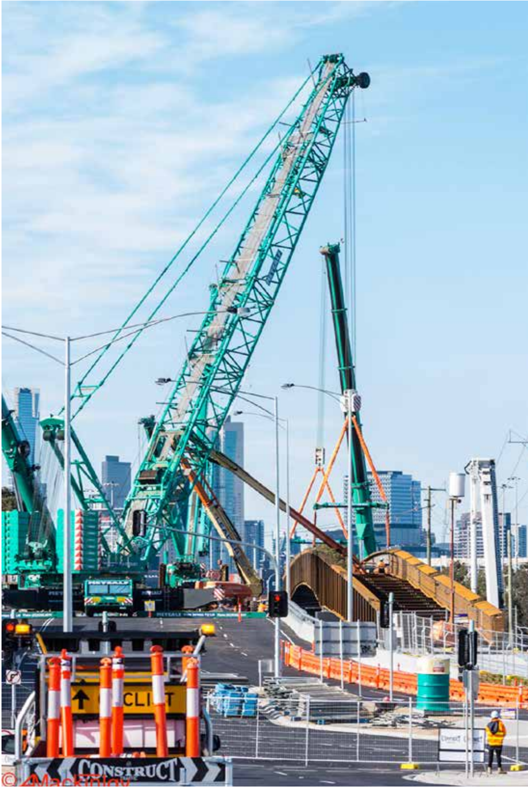
Stage 3: Steel sections E and F were spliced together on the ground and then lifted on to Pier 2 and spliced insitu to D. Stage 4: Steel section G connected to E-F and the east abutment to complete the main superstructure.
