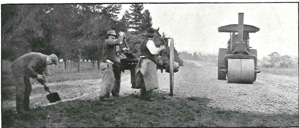
Plates 54 and 55. Showing earthy material and weeds being taken from water tables and spread on metalled roads.
