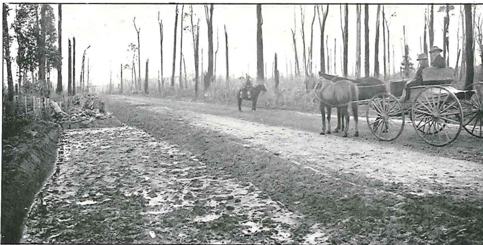
Plates 78, 79, and 80. Showing road works in Gippsland—Woorayl Shire. (1) Early stages of the work. (2) Contractor's portable stone-breaking plant. (3) Finished roadway.
