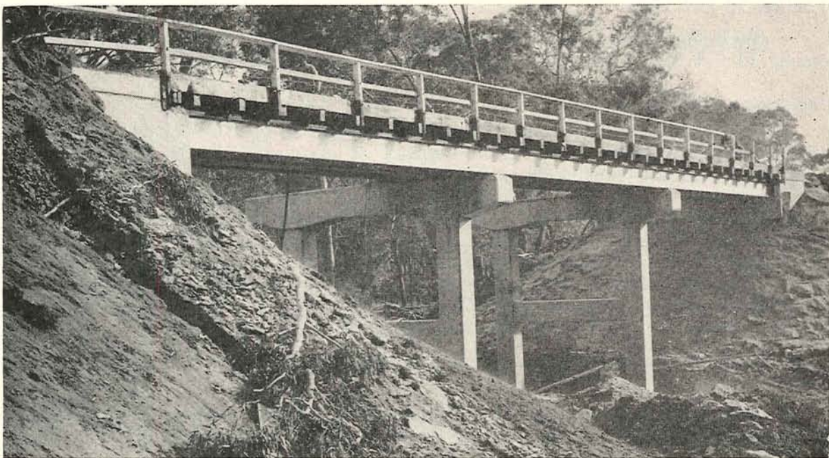
Plate 27.—Shire of Portland. Dartmoor—Hamilton Road. New bridge under construction over Crawford River.
