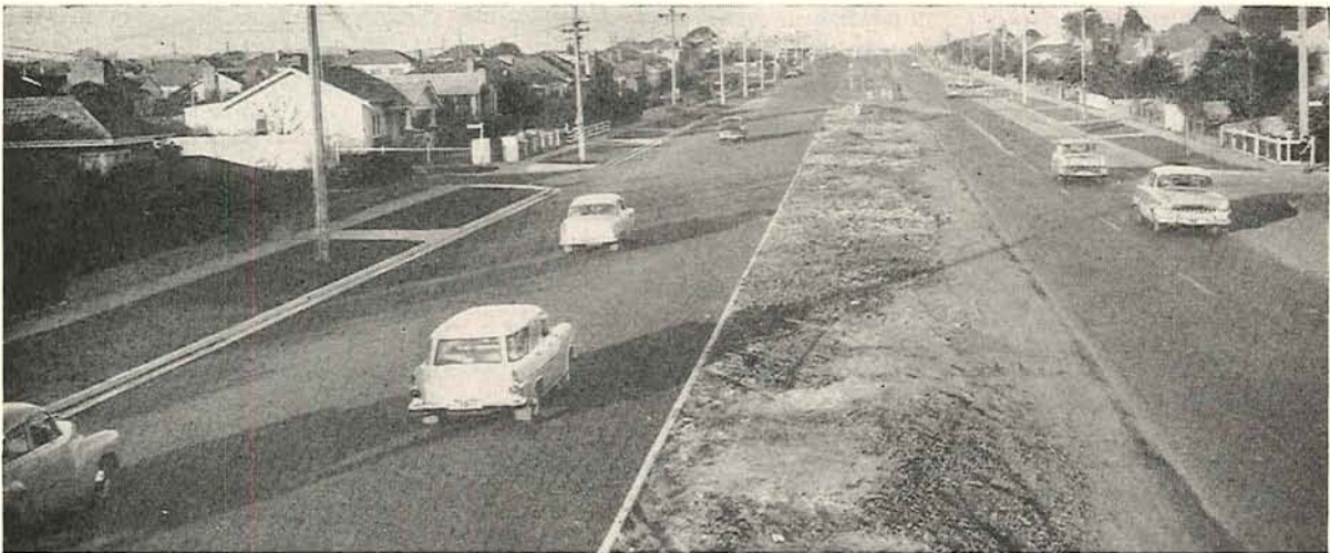
Plate 26.—City of Oakleigh—North Road. Duplication of pavement between Warrigal Road and Huntingdale Road.
