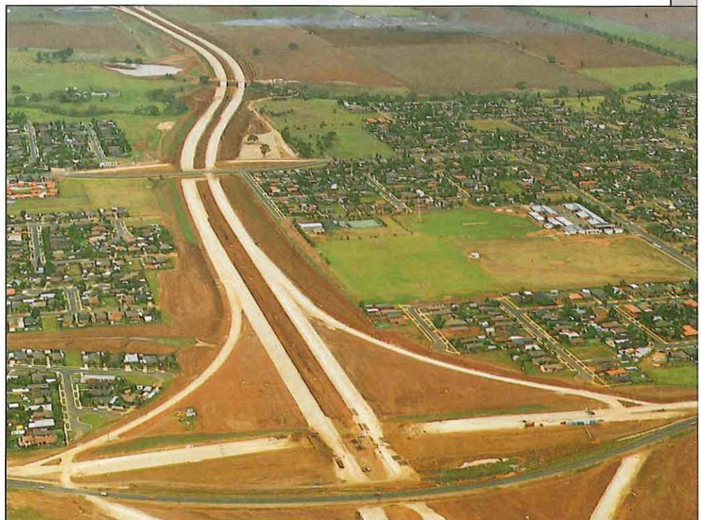
Western Freeway: construction of the Melton Bypass in progress, looking towards Melbourne
