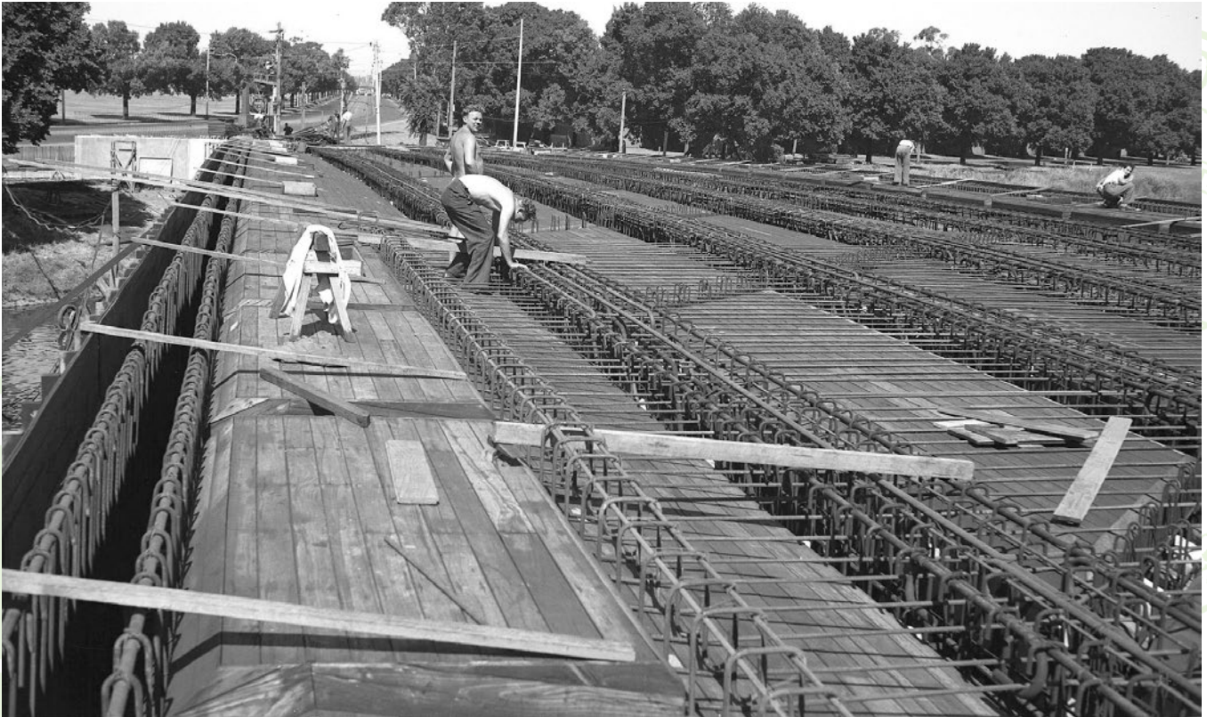
This photograph shows workmen placing reinforcement for the beams and deck of the bridge.
