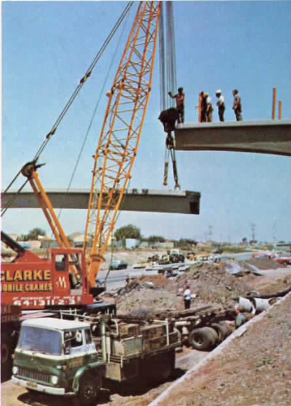
Placing the main span of the pedestrian overpass of the Calder Freeway at Niddrie
