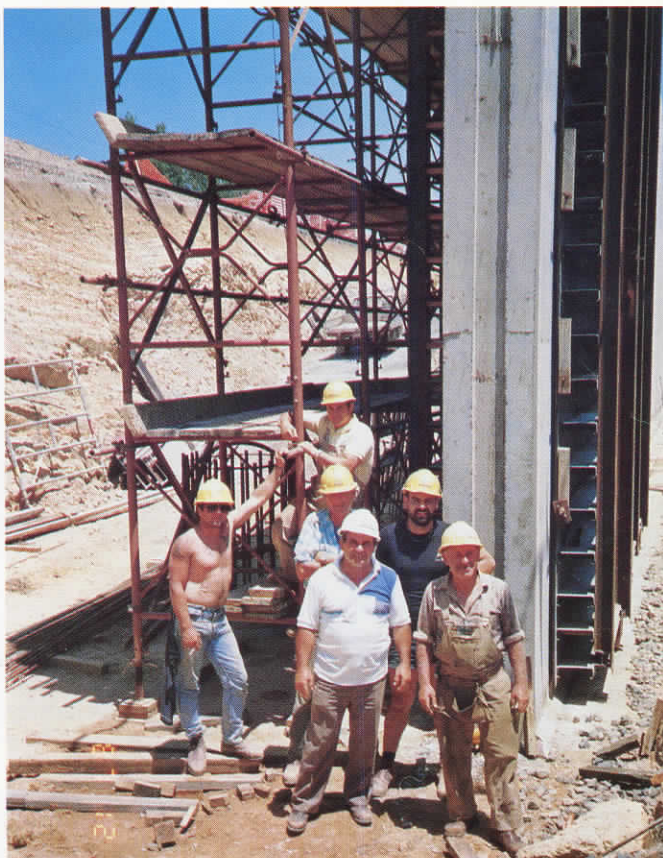
Sam Saccuzzo (front, centre) has high praise for the work of his bridge gang which helped develop the innovative trolley scaffold.
