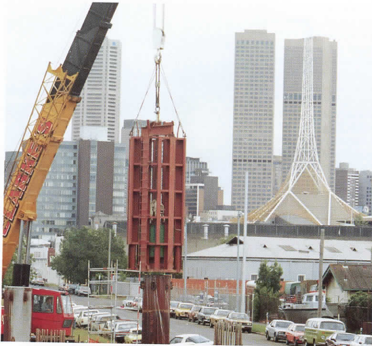
The hammer developed specifically for use at West Gate plunges onto a pile during a test.
