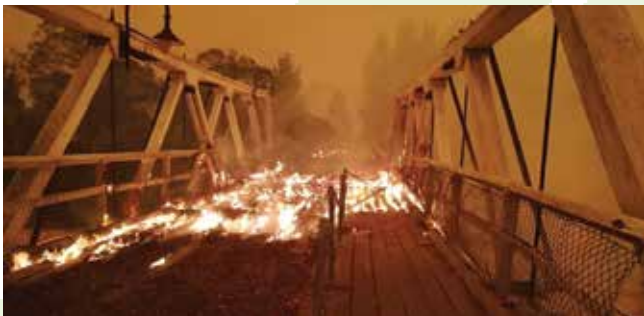
The deck of the Genoa River bridge caught alight.
