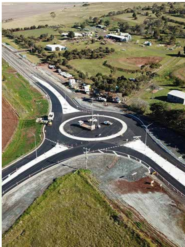
Construction of the roundabout at the Ballan Road and Parwan Exford Road intersection.
