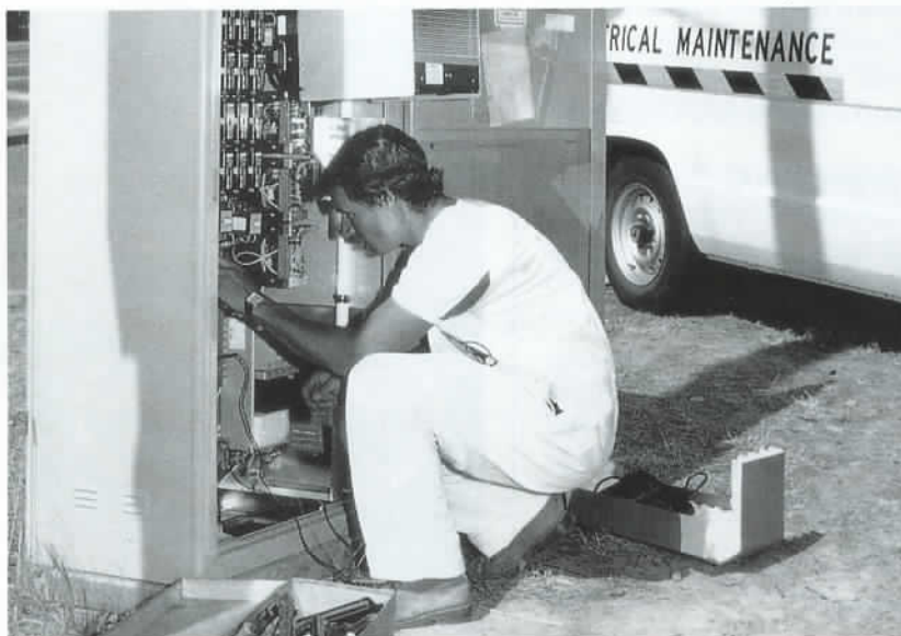
Traffic Signal Controller being installed by a VIC ROADS electrical maintenance worker.
