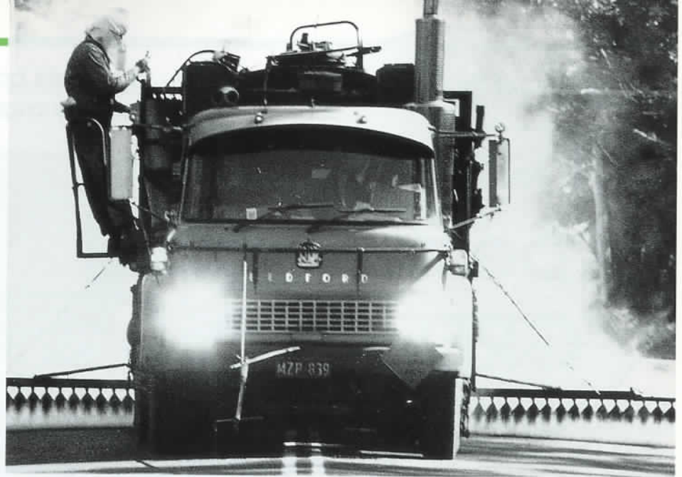
Summer is the time when VIC ROADS and municipal councils carry out resurfacing jobs on the road network. Drivers should always heed the advice of traffic controllers and warning signs at such sites.
