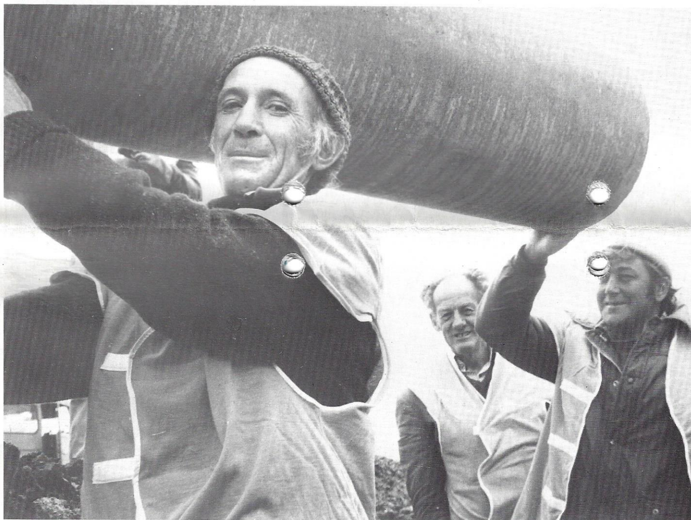
● Laying drainage pipes at Ballan are (from left) George Stewart, Leo Whitecross and John Dent.
