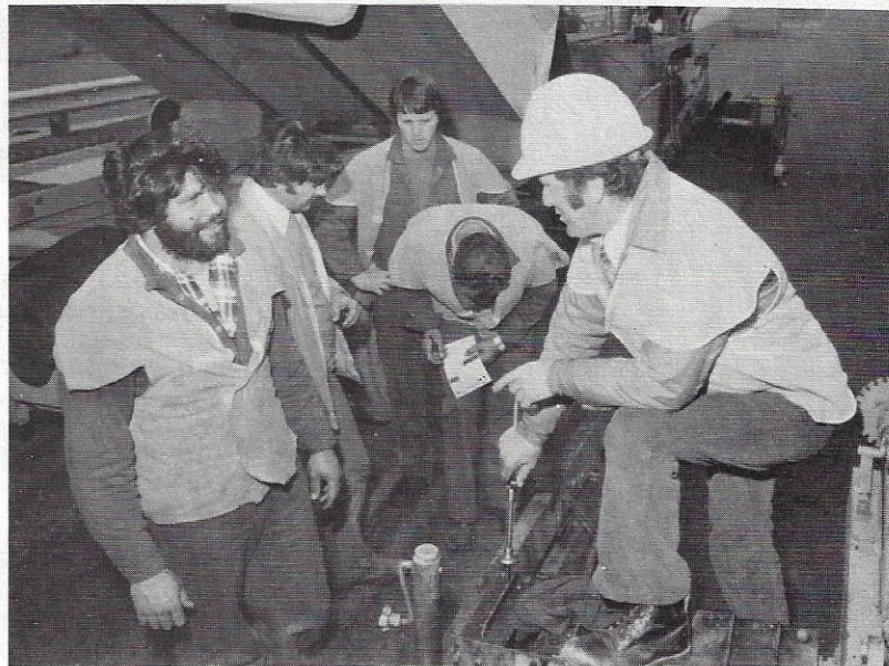
● Clerk of Works Gerry McLean (Metropolitan), right, discusses the asphaltting job with men on the job.
