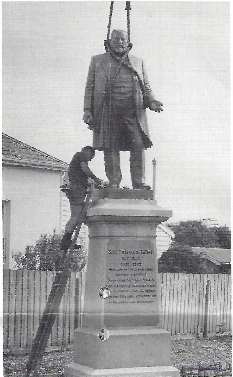
Sir Tommy was relocated by the CRB to his new landscaped site, at the corner of Hampton Street and the Nepean Highway, on Tuesday 25th March. He is pictured here, having just been lowered into place, being secured back onto his pedestal.
