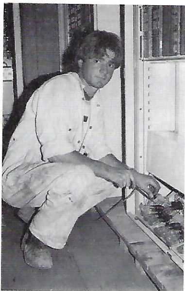
Above: John Mainie makes sure he's in the right circuits these days. He was presented with the third prize in the Electrical Apprentices Awards at Box Hill Tech recently. John, 20, works in the Electrical Installation and Maintenance section at Glen Waverley Depot.
