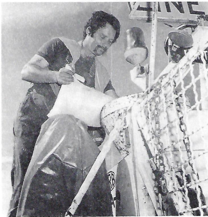
compressor which sprayed paint from a 16 gallon container. Today the CRB employs about 70 men who are involved in maintaining the system of linemarking, road markings and raised pavement markers throughout the State.
