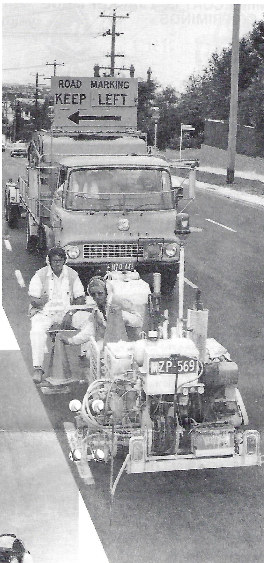
Linemarking Latrobe Terrace in Geelong are overseer Mel Pike (left) and operator Karl Fraatz. Brian Ried is following in the escort truck.
