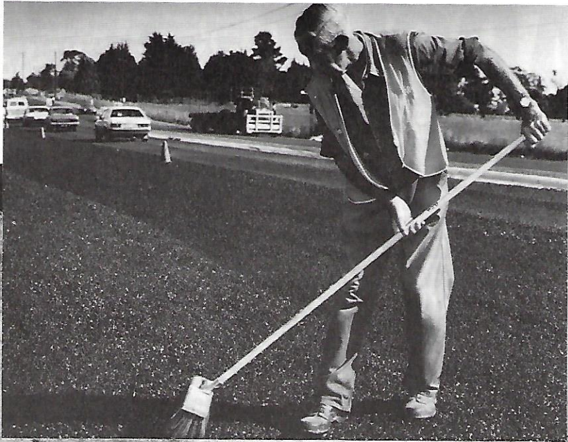
Left: Making a clean sweep of things. Stan Moyle spreads excess aggregate to ensure an even distribution on the road surface. Below: The sprayer has just started its run as Sprayer Operator, Ernie 'Tube' Hade, releases the controls and bitumen is sprayed onto the road. Malcolm Sandy (left), Peter 'Kojak' Kaljouw and Peter 'Billygoat' Middleton prepare to remove the starting papers. Most of the crew have been bestowed with nicknames.
