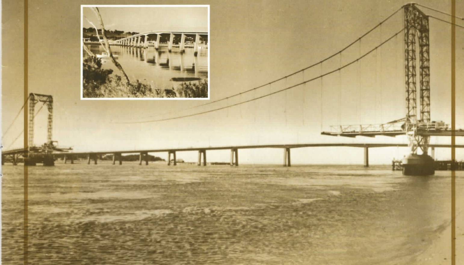
Dismantling of the old Phillip Island suspension bridge, 1969. Inset : the bridge today
