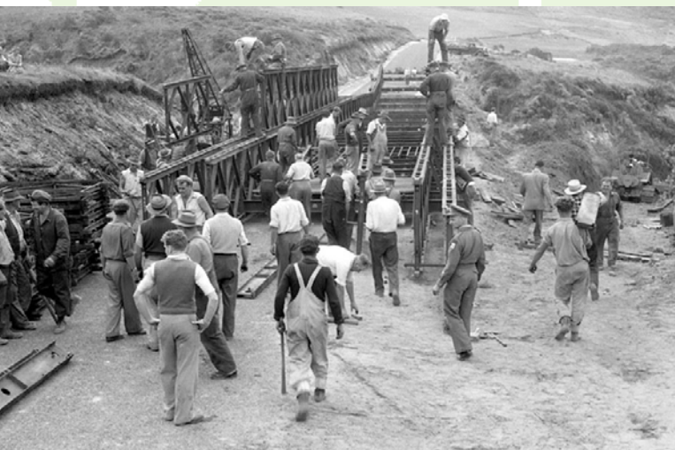
Assembling the Bailey bridge. Alec is standing in the foreground in the sleeveless sweater. Note the presence of Army personnel. I suspect the bridge panels belonged to the Army.
