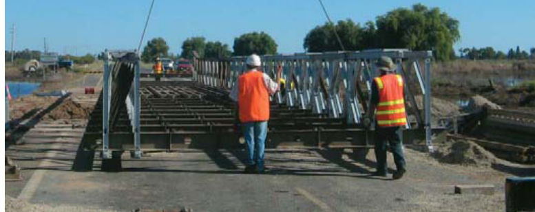
The teams at Northern and Western Regions and SprayLine Road Services assembled a "Bailey bridge" near Kerang.
