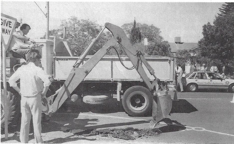
The Minister on site at the 32nd blackspot treatment site in Mildura.
