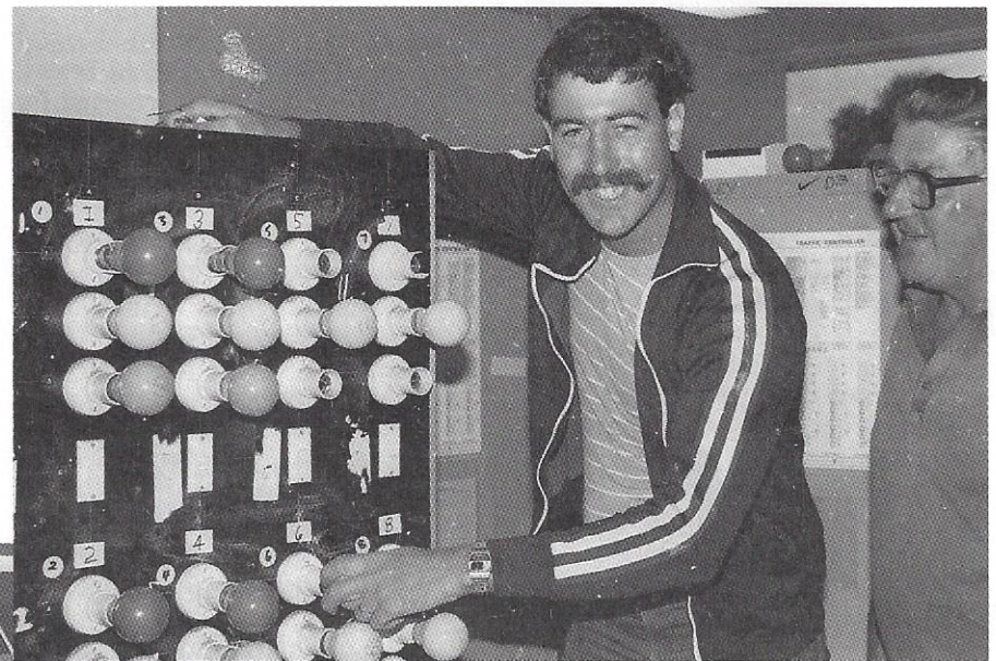
Traffic Signal Technician Stu Hamilton and Jim Howard - both recently transferred from MCC - changing lamps in a mimic panel.
