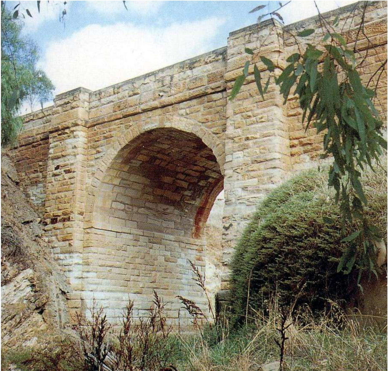
Figure 4.3 The 1859 Djerriwarrh Creek Bridge on the Old Western Hwy at Melton CRB
