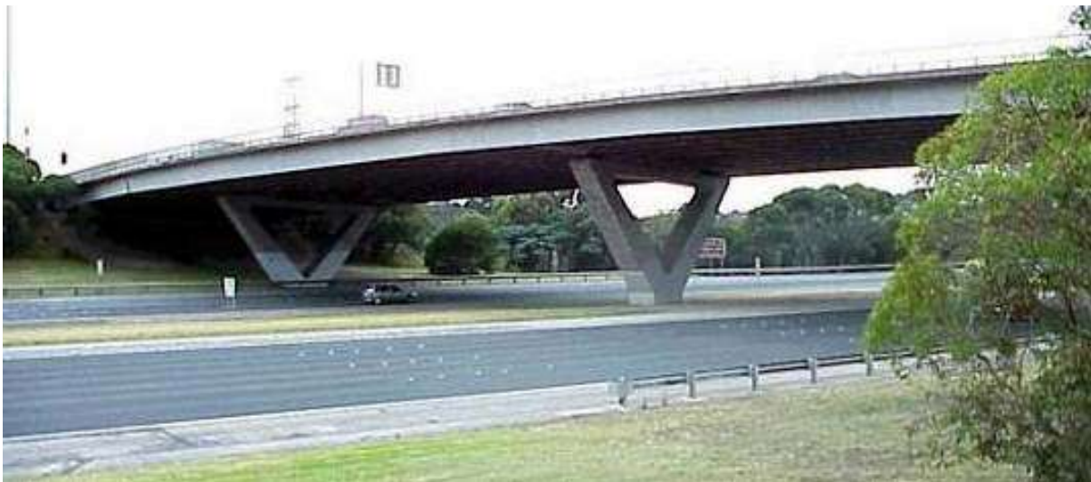
Figure 6.3 Fine lines of the Burke Rd bridge over the Eastern Freeway, looking east.
