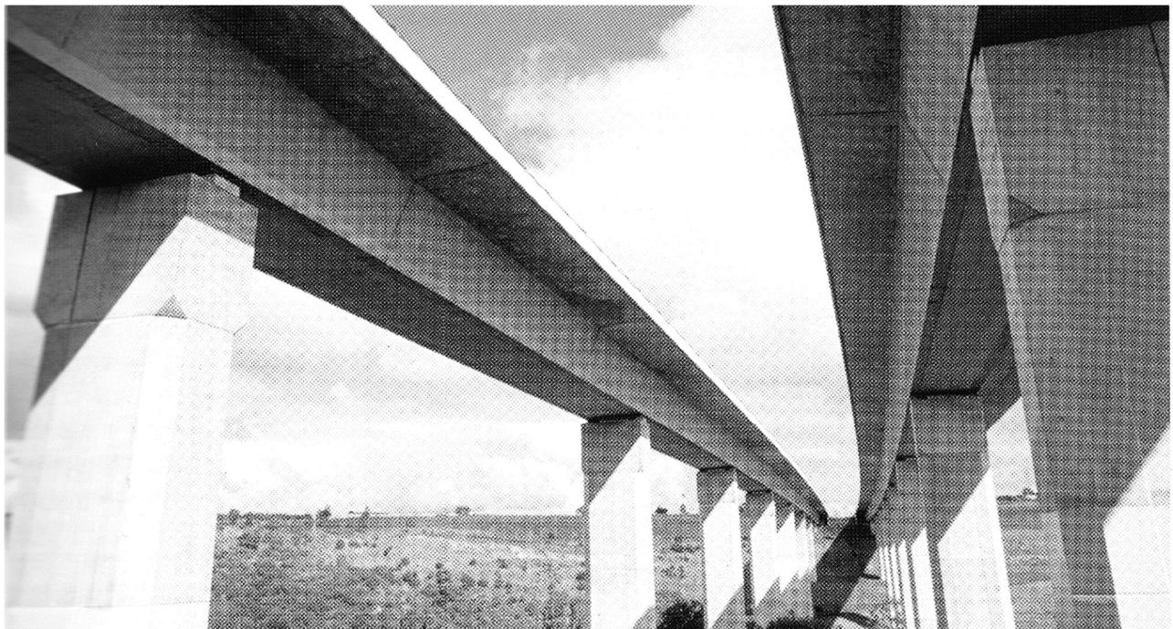
Figure 6.2 The E J Whitten bridge over the Maribyrnong River at completion in 1995 VicRoads Annual Report, p4
