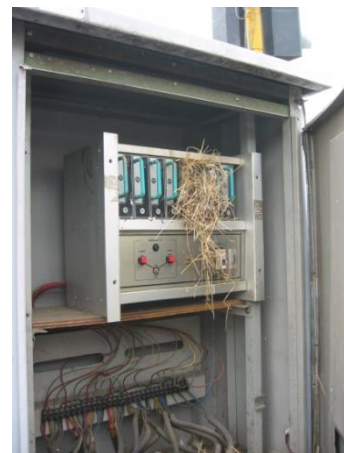
Bird nest in signal control cabinet, Medan North Sumatra
