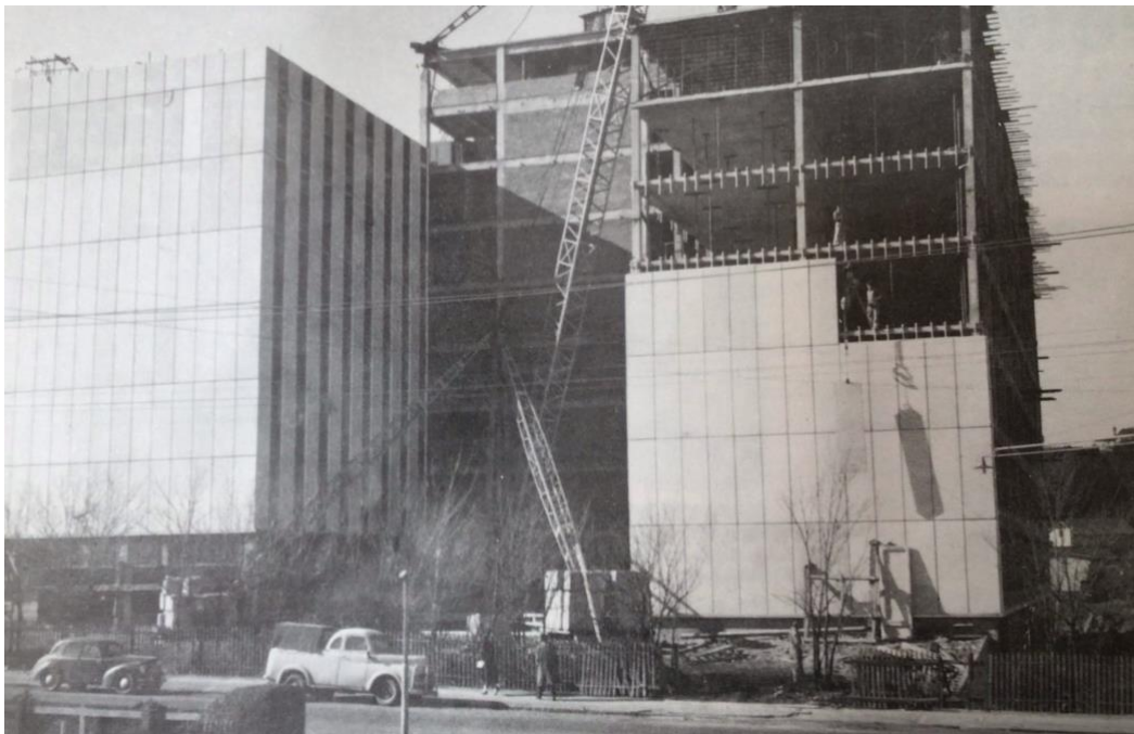
The same view showing the external cladding being placed. It looks as if the ute was permanently parked in Denmark Street.
