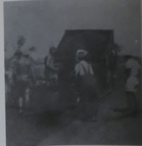
• No bulldust—it's hot work! Men spreading a bitumen wearing course on Stuart Highway near Tennant Creek
