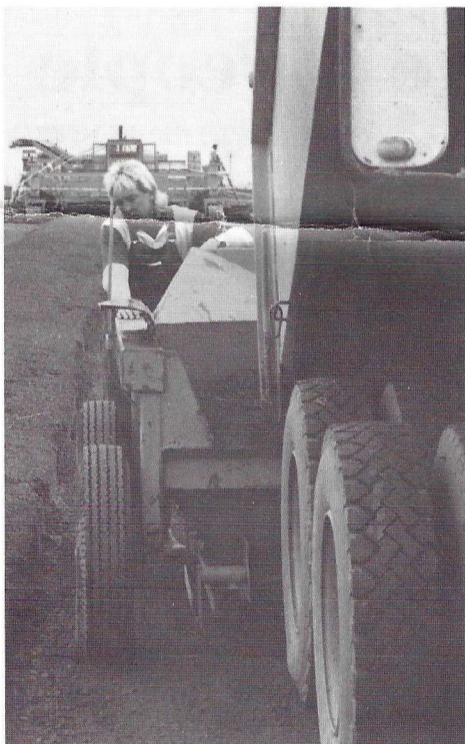
• Andrew Attwell operating the windrow box. The crushed rock is wet mixed at a plant on site, delivered to the roadbed, and tipped onto the road through the 'windrow box'.
