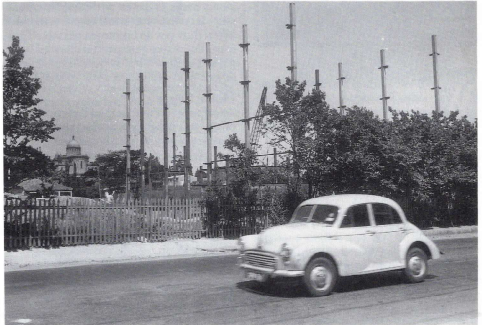
■ Above: A Morris Minor speeds past the rising scaffold for Victoria's new roads headquarters.
