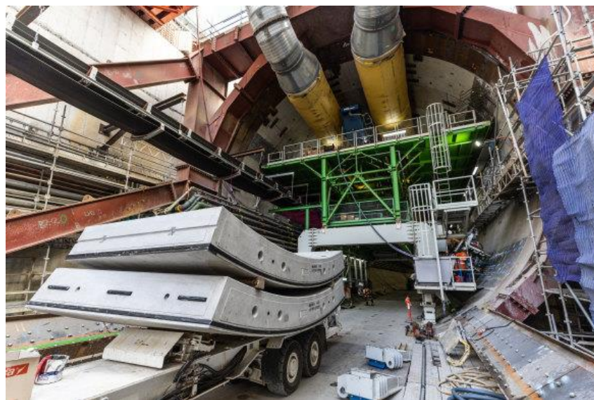
The entrance to one of the tunnels with precast concrete liner segments in the foreground.
