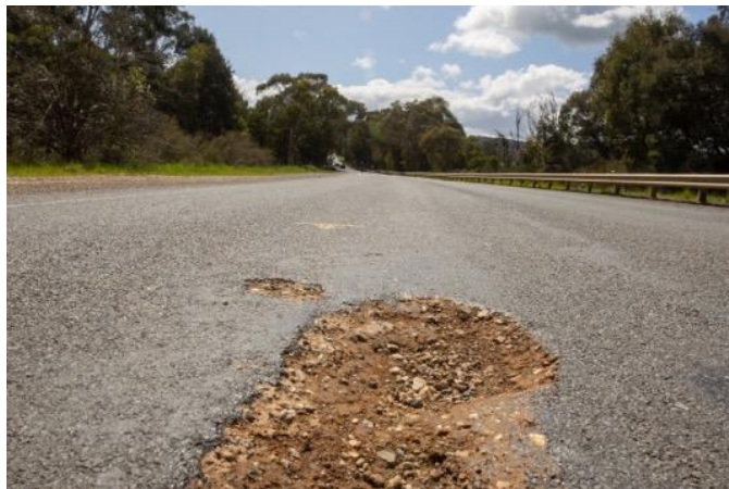
A pothole on the Melba Highway.
