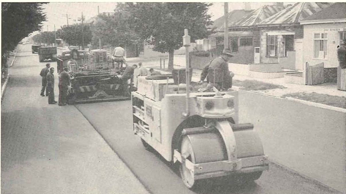
Plate 6.—Ballarat Road near Rosamond Road. Channels reconstructed and asphalt laid, City of Sunshine.
