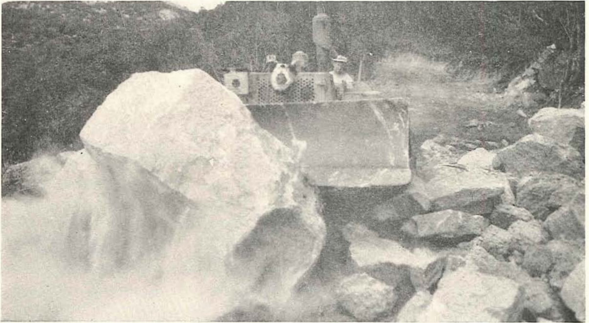
Plate 13.—Shire of Bright. Mt. Buffalo Road (The Horn section). Widening in progress south of the Cathedral.
