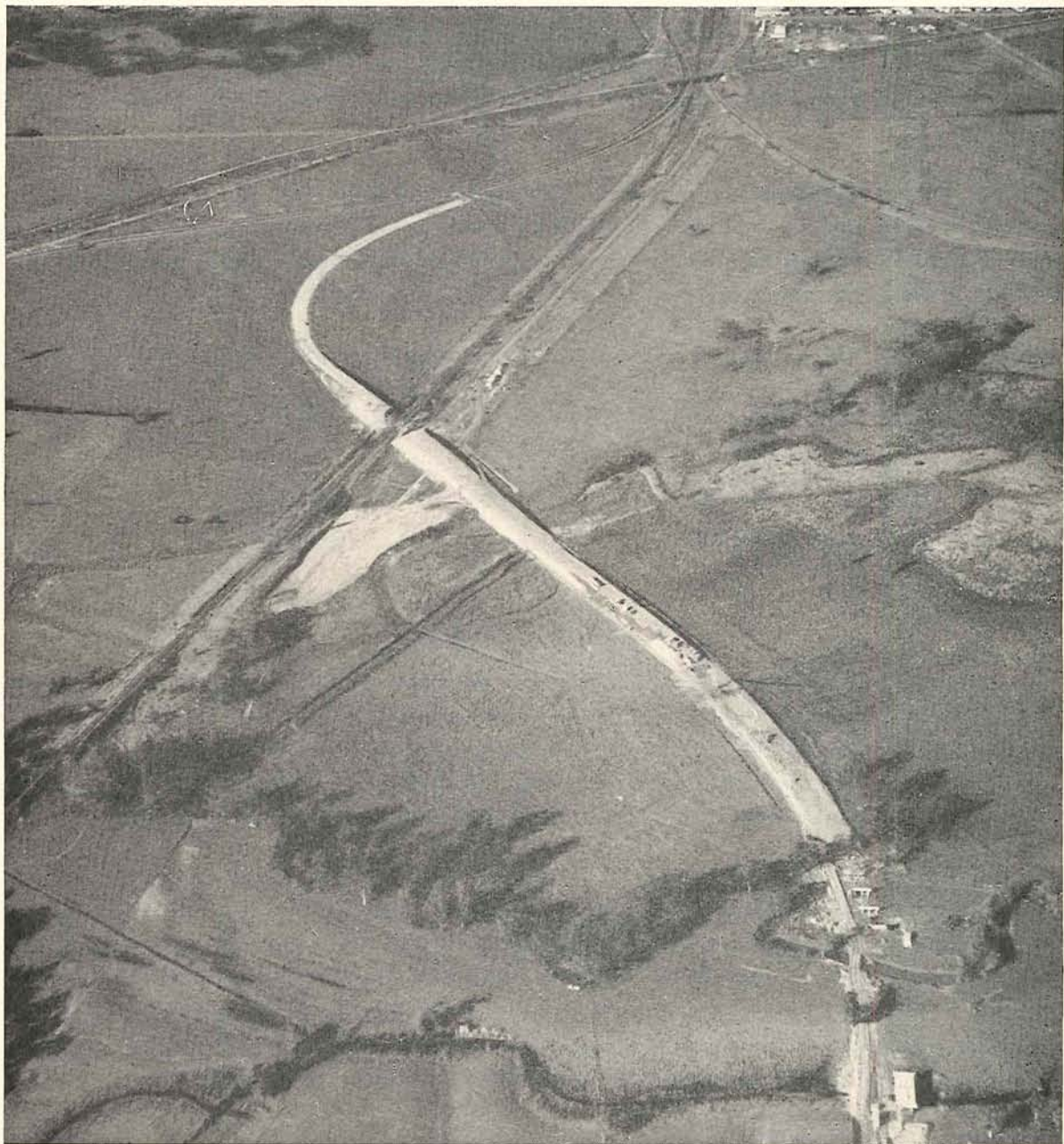
Plate 44.—Princes Highway East. Realignment under construction between Herne's Oak and Morwell, looking towards Morwell.
