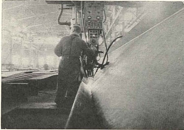
Plate 10.—Welding a girder flange to the web using a single head, fully automatic machine.
