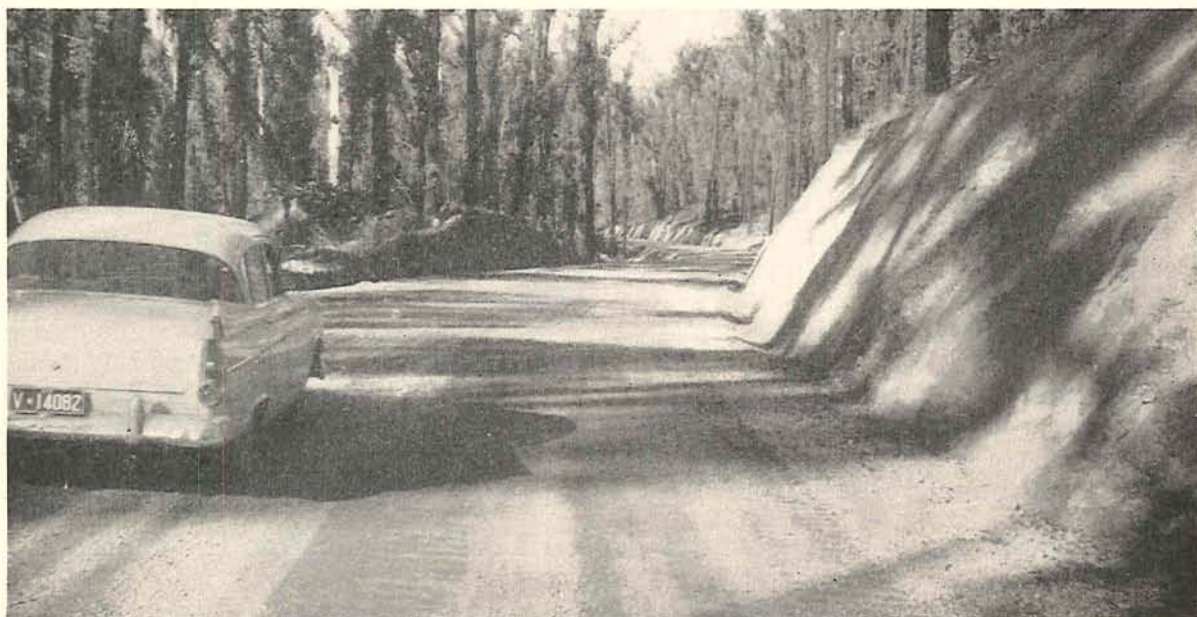
Plate 21.—Shire of Orbost. Club Terrace Loop. Section constructed by contractor on new alignment near Bemm River, Princes Highway East.
