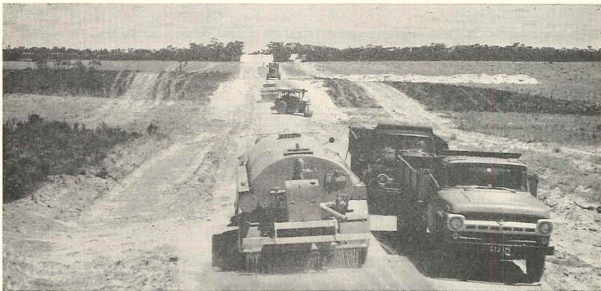
Plate 43.—Shire of Kaniva. Serviceton North Road. Big Desert Area. Spreading and consolidating sandstone pavement.
