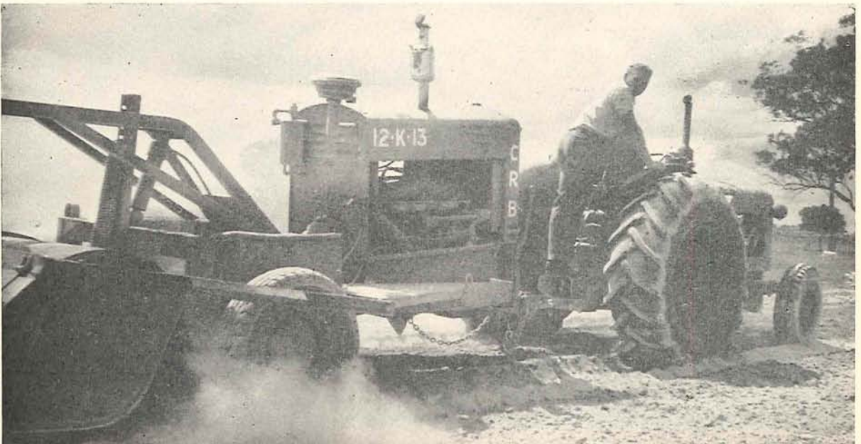
Plate 29.—Murray Valley Highway, Section 2, 132.46 to 138.88 miles. "Seamen" pulverizer being used for final mix.
