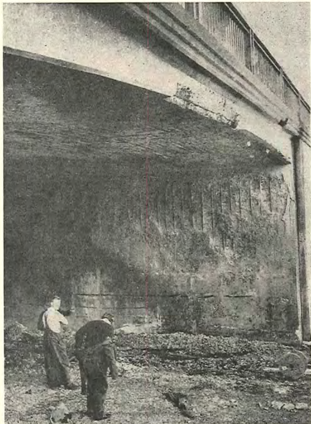
Plate 6.—Shepherd Bridge. General view of the upstream section, showing spalling damage caused by fire.
