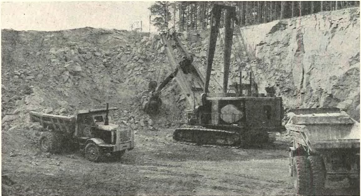
Plate 2.—Special Project No. 7. Heavy rock work in the cutting near Pykes Creek on the Western Highway.
