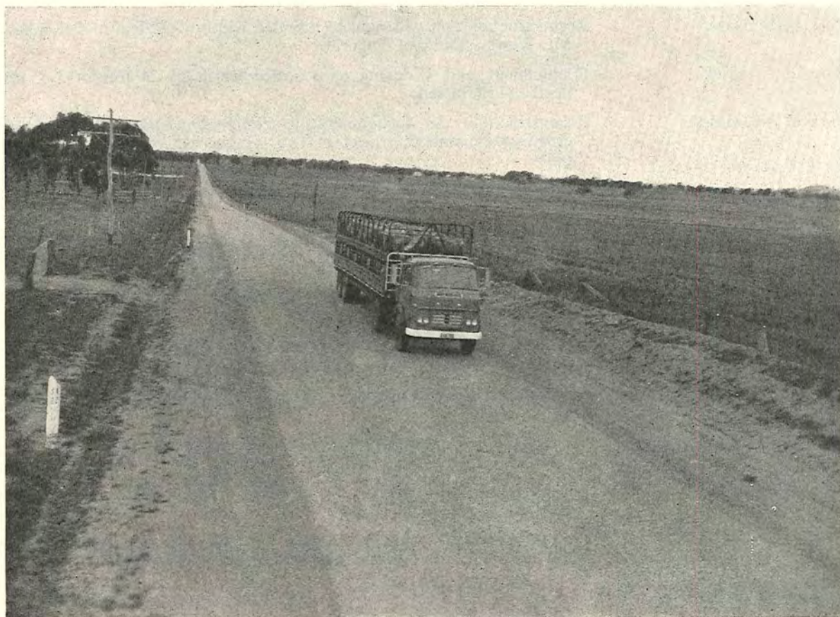
Plate 35.—Wimmera Highway—widened and resheeted section between Marnoo East and Boyles Bridge—Shire of Kara Kara.
