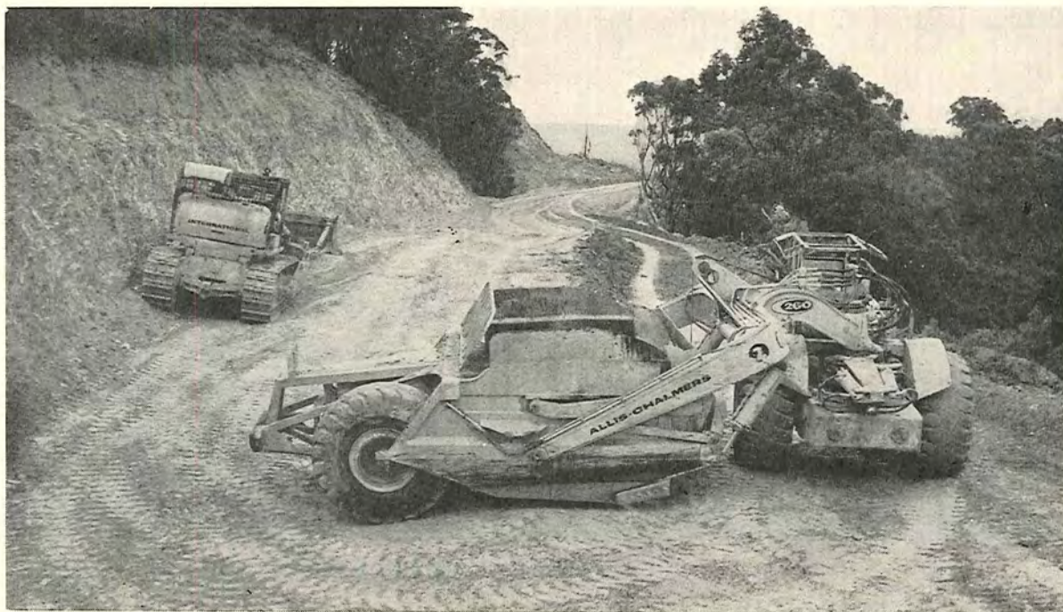
Plate 14.—Contractor's plant in operation on the Foster deviation—South Gippsland Highway—Shire of South Gippsland.
