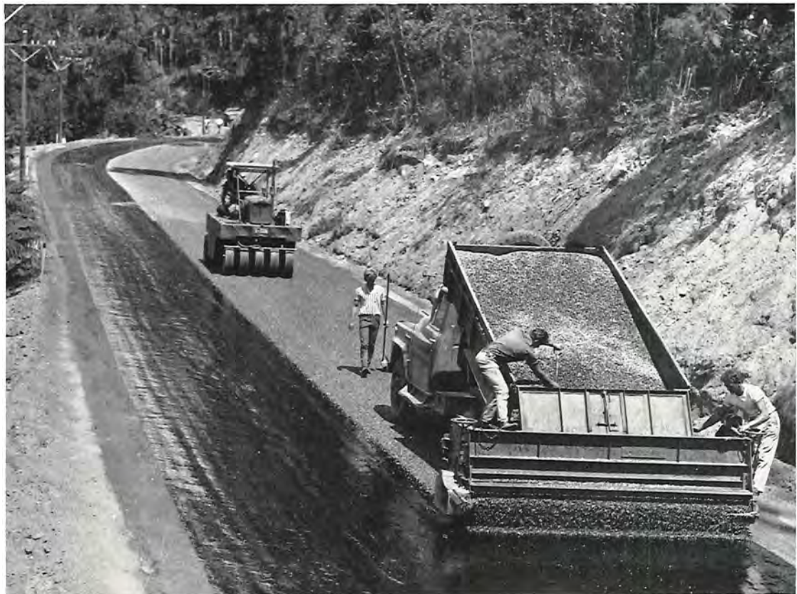
Completing the bituminous sealed pavement between Melbourne and Sydney on the Princes Highway East near Mount Drummer.
