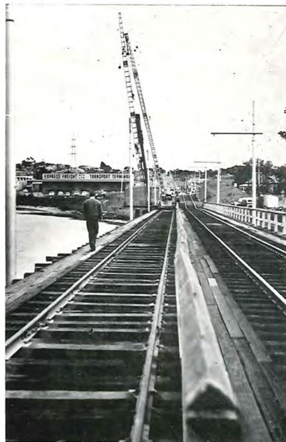
Plate 1—Maribyrnong River Bridge, Raleigh's Road. General view showing limited working space available for pile driving frame.
