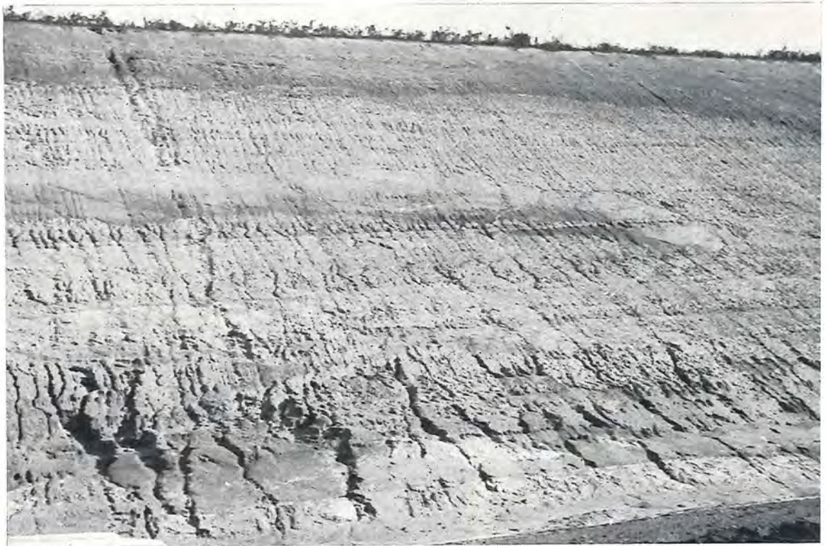
Plate 1 — Batter Stabilisation, Princes By-pass Road, Moe. Erosion Effects on Unstabilised Batter before Treatment.
