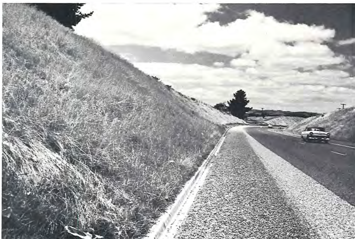
Plate 2 — Batter Stabilisation, Princes By-pass Road, Moe. Cover Growth for Stabilisation after Treatment.
