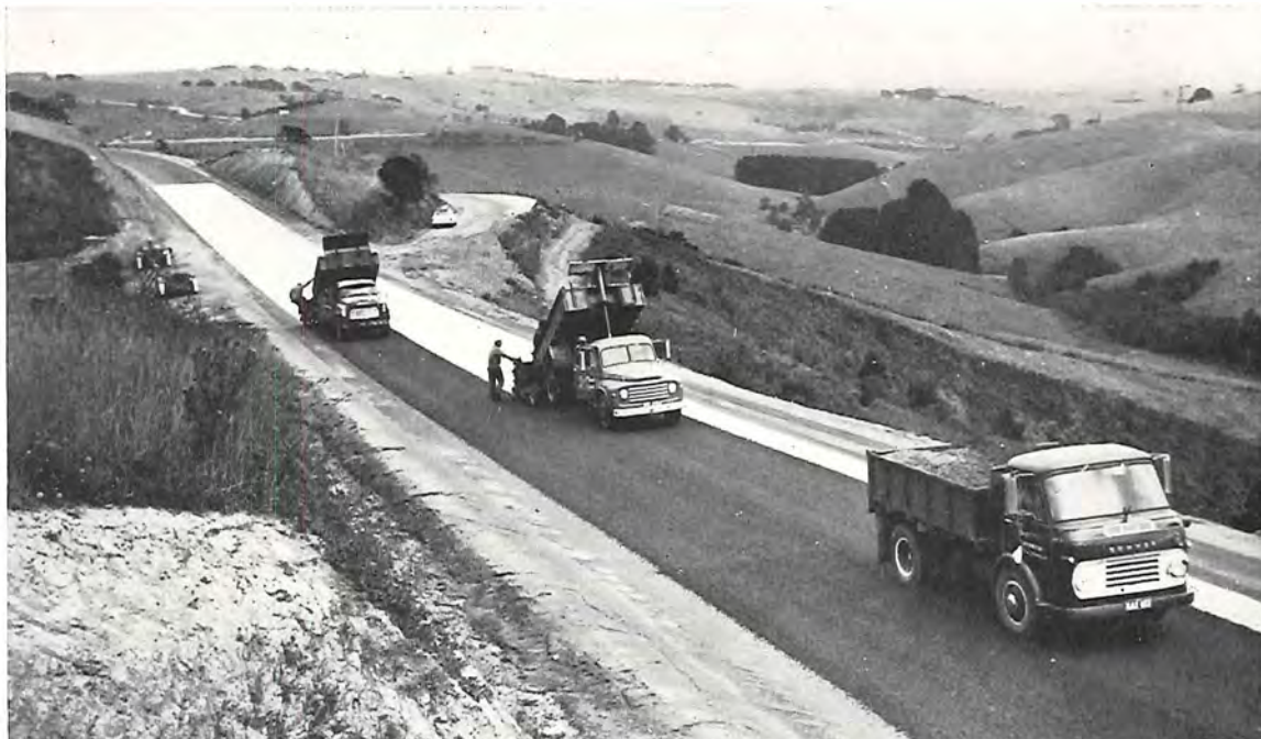
South Gippsland Highway, Shire of South Gippsland. Sealing in progress north of Foster.
