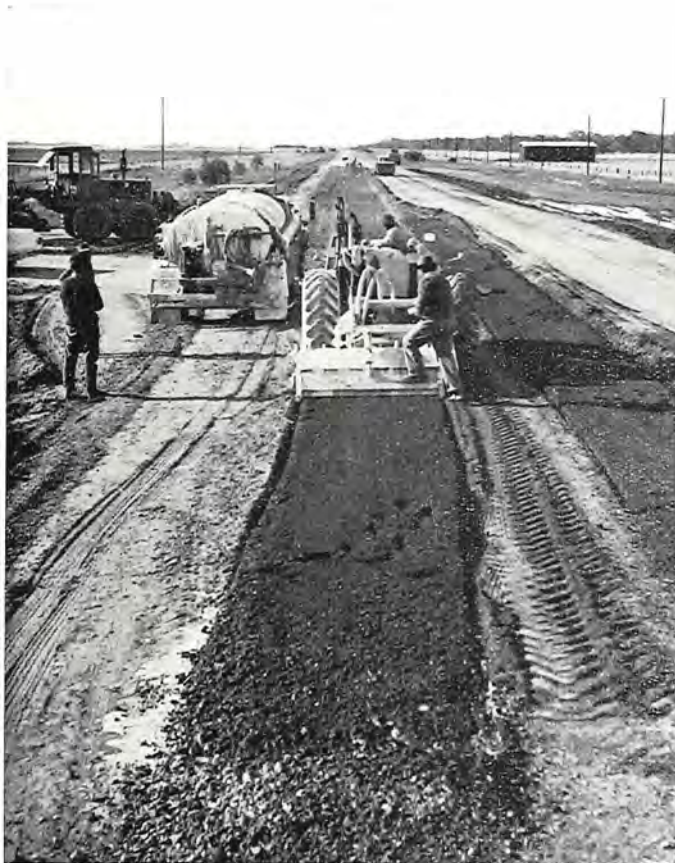
Northern Highway, Shire of Rochester. Reconstruction with lime stabilisation north of Rochester.
