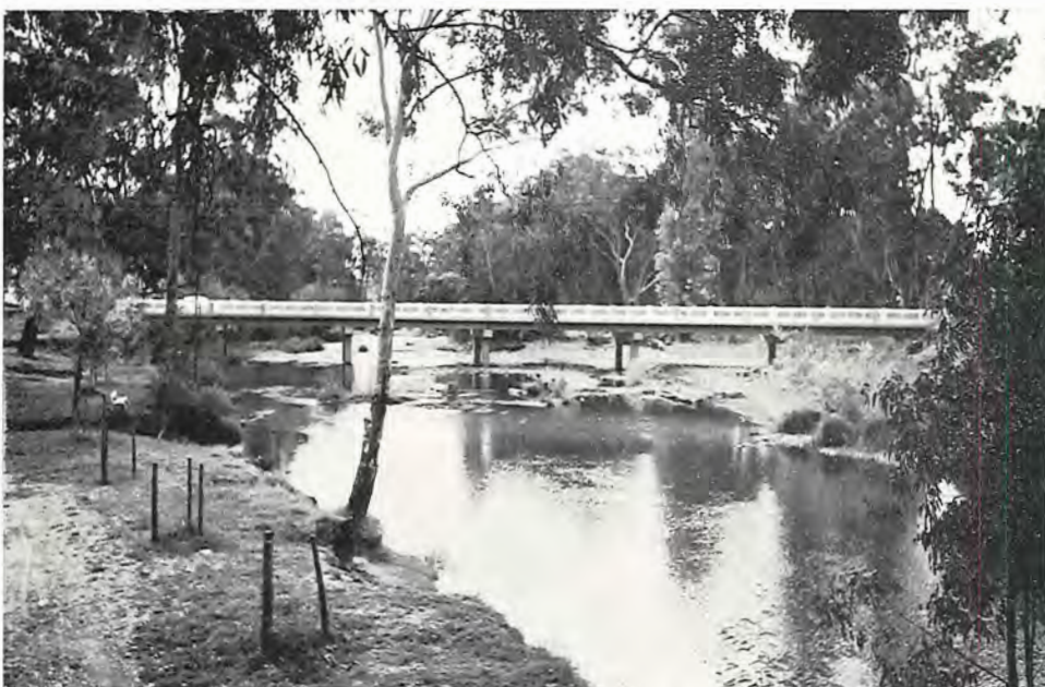
New bridge over the King River on the Edi-Cheshunt Road, Shire of Oxley.
