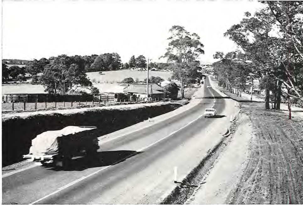
Princes Highway East, Shire of Buln Buln. Reconstruction and realignment between Robin Hood and Drouin.
