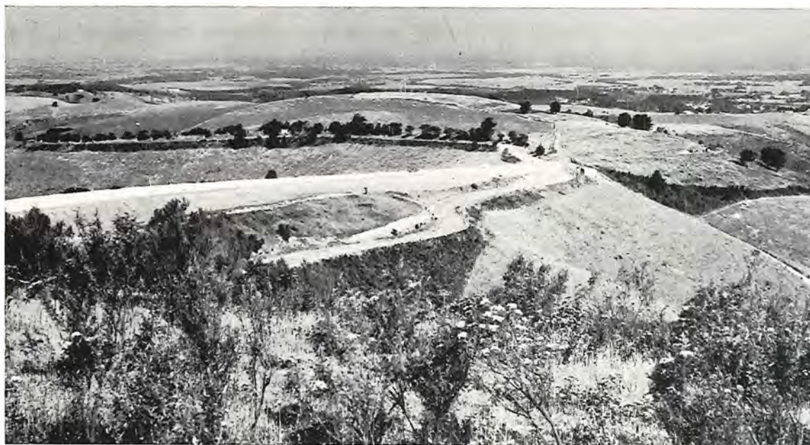
South Gippsland Highway, Shire of South Gippsland. Reconstruction on an improved alignment north of Foster.
