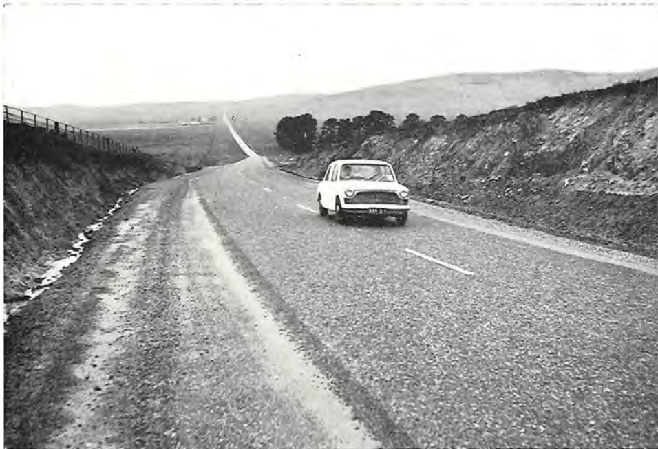
Benambra Road, Shire of Omeo. Reconstruction to provide a sealed pavement 12 feet wide.
