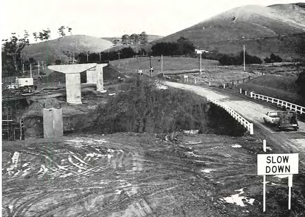
South Gippsland Highway, Shire of Korumburra. Construction of an overpass of the south-eastern railway line and Alsops Creek.
