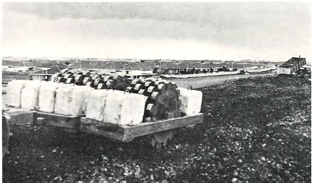
Plate 7—Forty ton static tamping roller, used in compacting Lower Yarra Freeway embankments.
