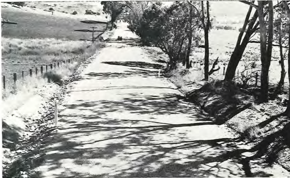
Tallangatta Creek Road, Towong Shire. Reconstruction to provide a sealed pavement 18 feet wide.
