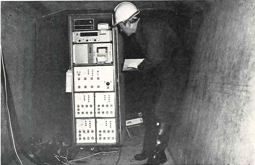
Plate 2—Bell Street Bridge, Automatic recording equipment used during the structural research programme.
