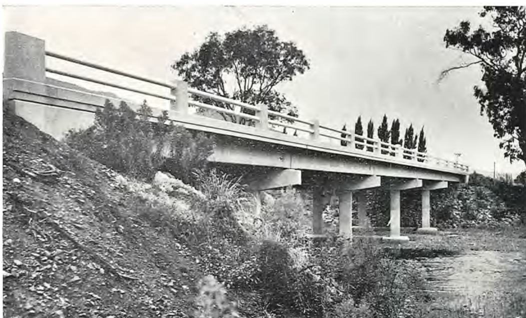
Buffalo River Road, Myrtleford and Oxley Shires. Bridge over Buffalo River (McGuffies Bridge).
