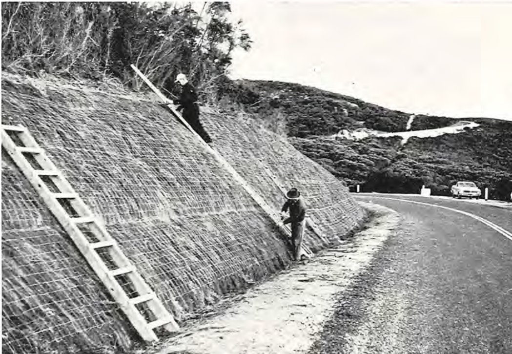
Batter treatment on Wilsons Promontory Road south of Darby River.
