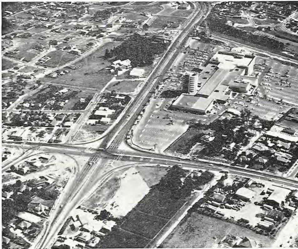
Doncaster Road, Doncaster and Templestowe City. Reconstruction at intersection with Heidelberg-Doncaster Road.
