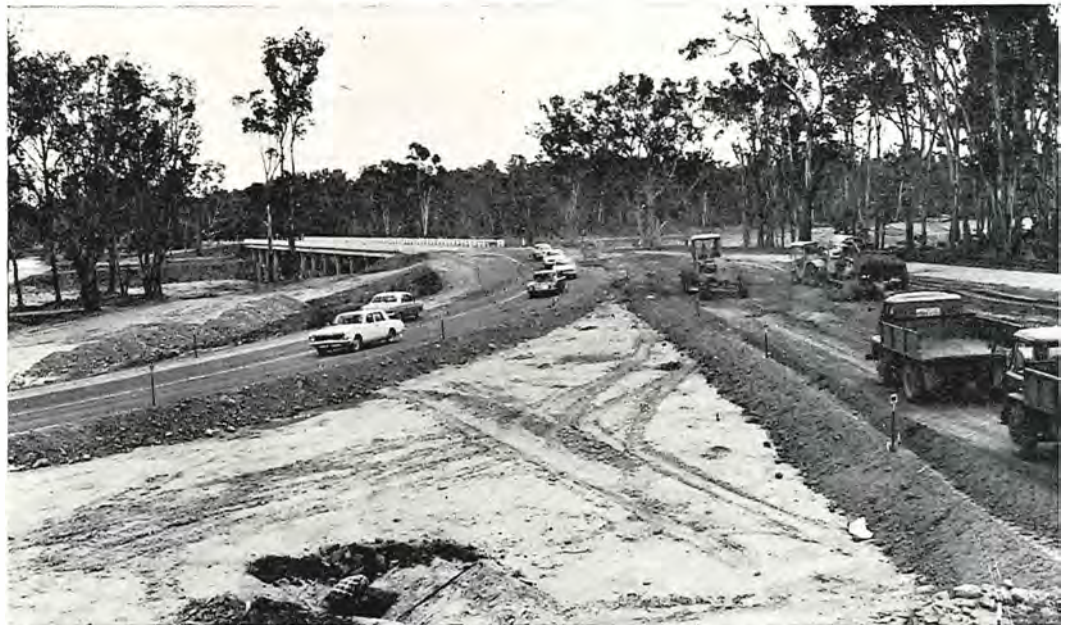
Construction of new approaches to Shepparton at Bridge No. 2 on the Midland Highway.
