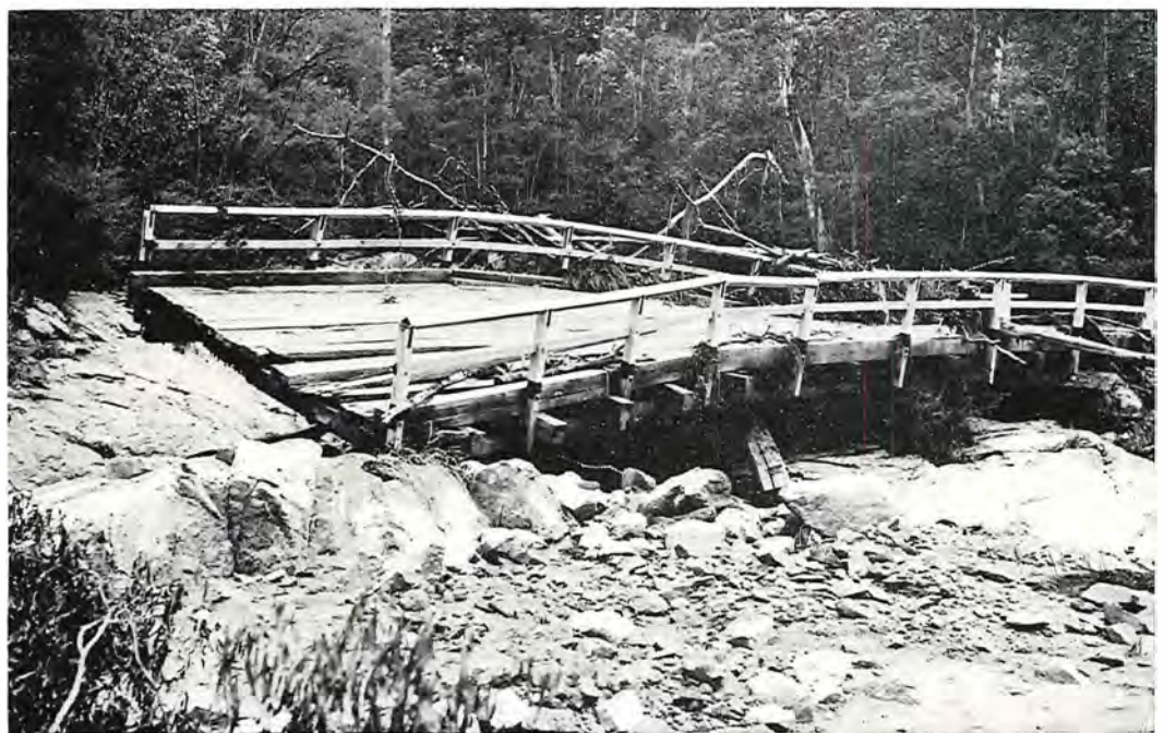
Bridge at Winnets Creek on the Cann Valley Highway damaged by floods.
