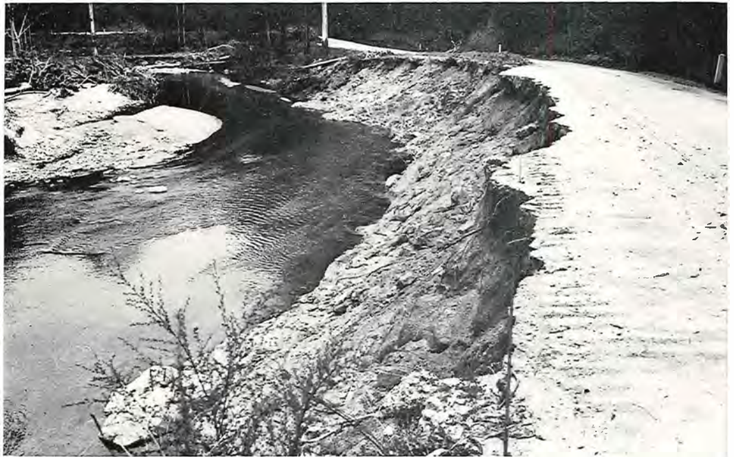
Flood damage to the Cann Valley Highway 16 miles north of Cann River.
