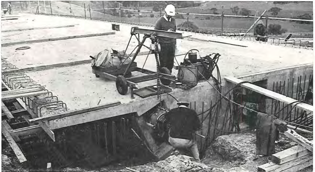
Construction of the western interchange bridge on the Western Freeway (Bacchus Marsh section).
