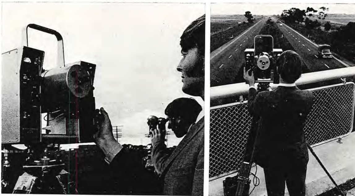
Plates 8 and 9—Use of the Board's Geodimeter 6A electronic distance measuring equipment during a project control survey.
