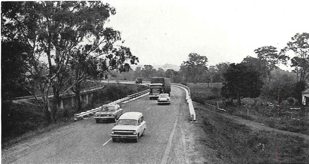
Reconstruction of the Goulburn Valley Highway on a new alignment near Molesworth.
