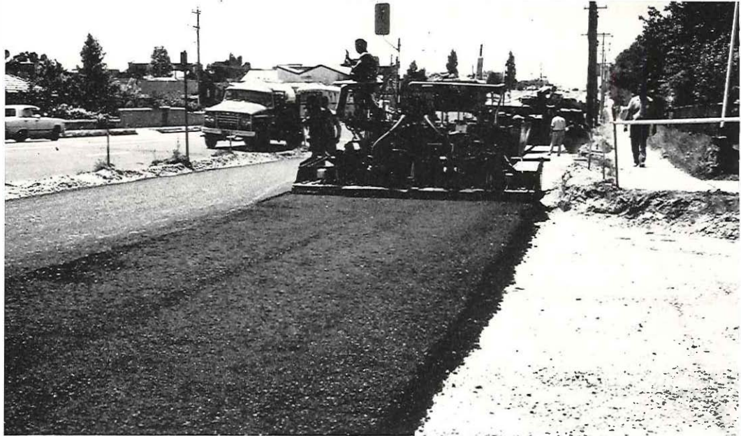
Plate 12—Springvale Road in Waverley City under construction with a deep strength asphalt pavement. The first 4 in. layer of asphalt is being placed on a 6 in. lime stabilized clay subgrade.
