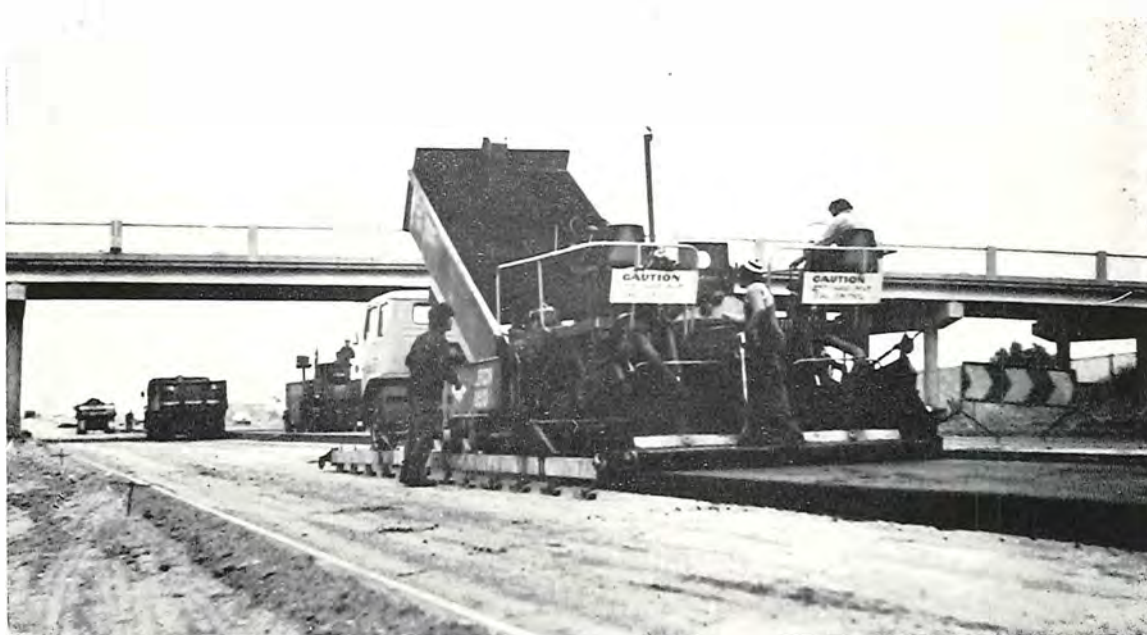
Plate 16—Placing full depth asphalt widening straight on to a prepared sub-grade on the Princes Highway West
