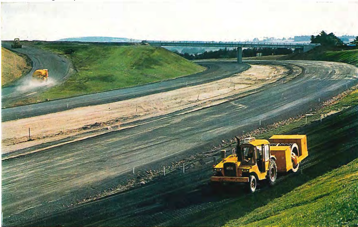
Work in progress at the Greendale interchange on the Western Freeway (Myrning Section).
