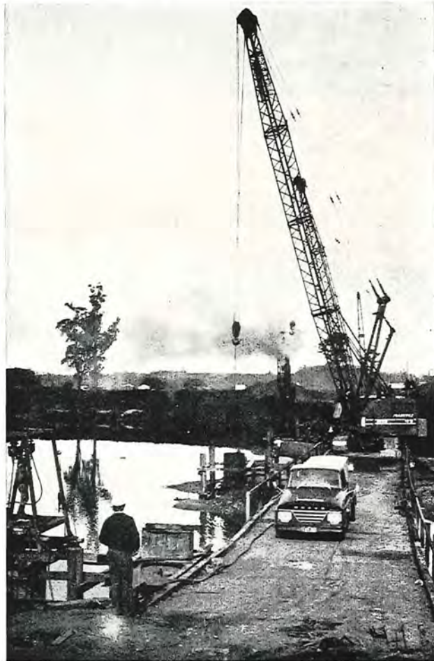
Plate 3—Driving and cleaning out steel cylindrical piles for the piers in the main river channel.
