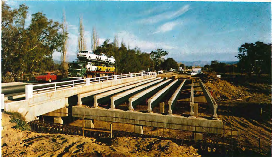
Providing for dual carriageways on the Lincoln Causeway (Hume Highway) between Wodonga and the Murray River
