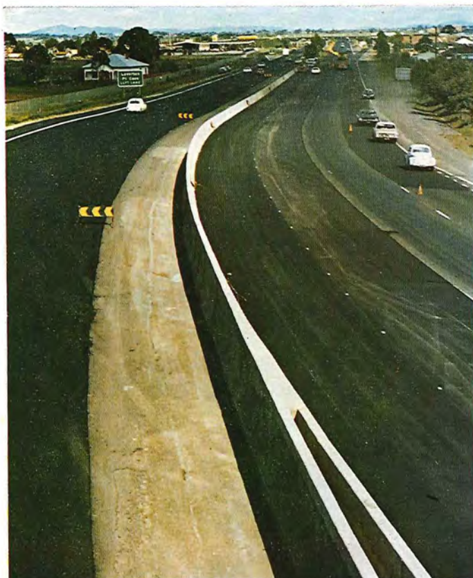
Section of median barrier wall built along the Princes Freeway near Laverton.
