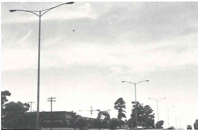
Plate 12: Street lighting installation on the Princes Highway East in the City of Springvale.
