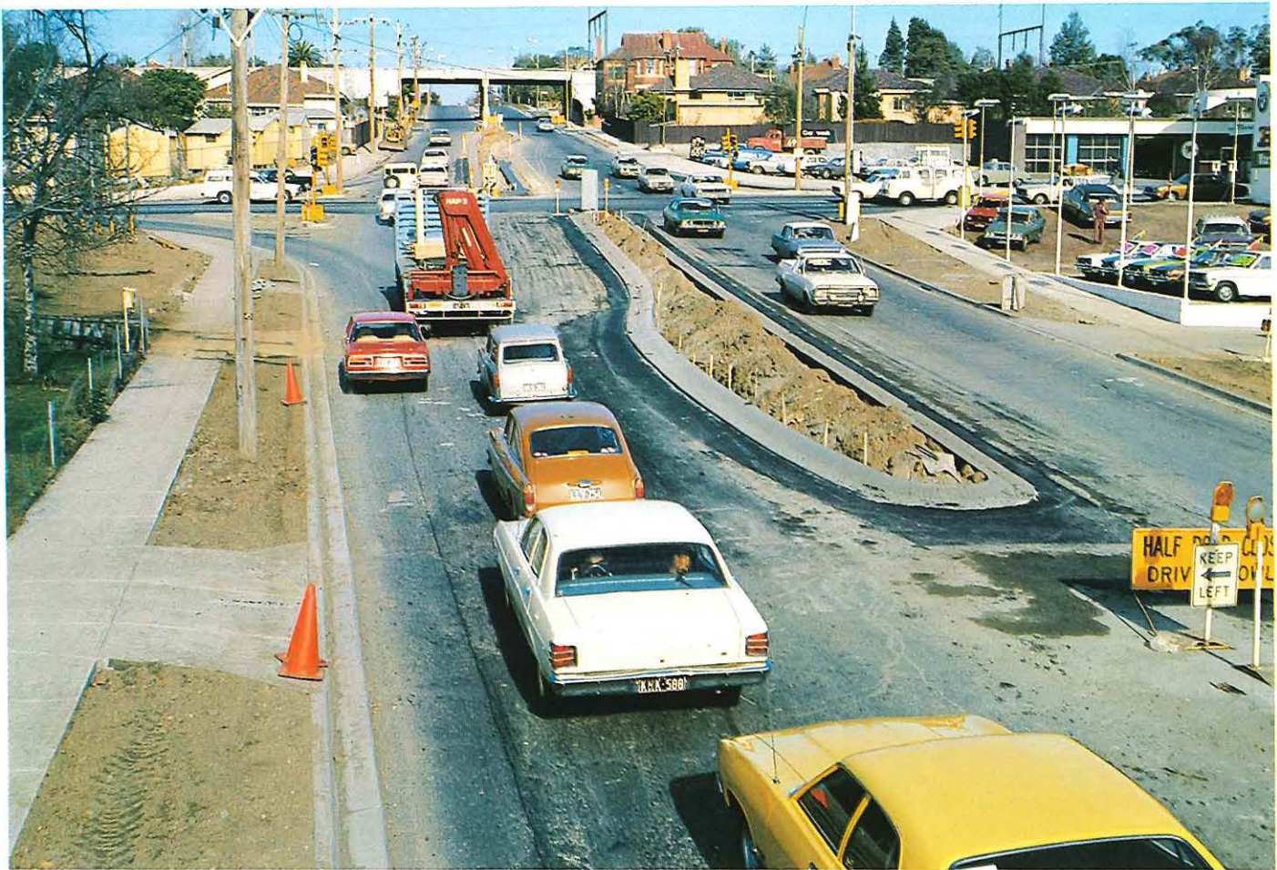
Intersection improvements provide safer roads. Top, Lower Heidelberg Road and Banksia Street, Heidelberg; Below, Maroondah Highway and Elgar Road, Box Hill.
