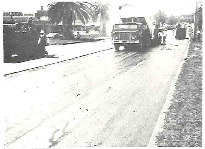
Plate 9: Placing of coarse graded asphalt containing scrap rubber granulate. Nepean Highway, Mordialloc
