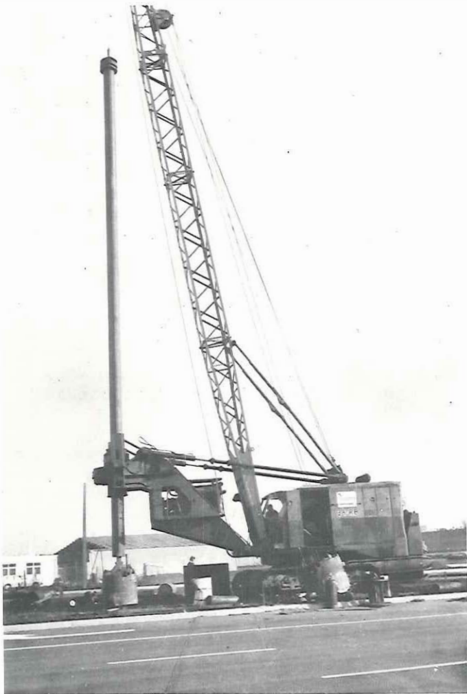
Plate 8: TG 200 rotary drilling rig used for the excavation of the steel casings
