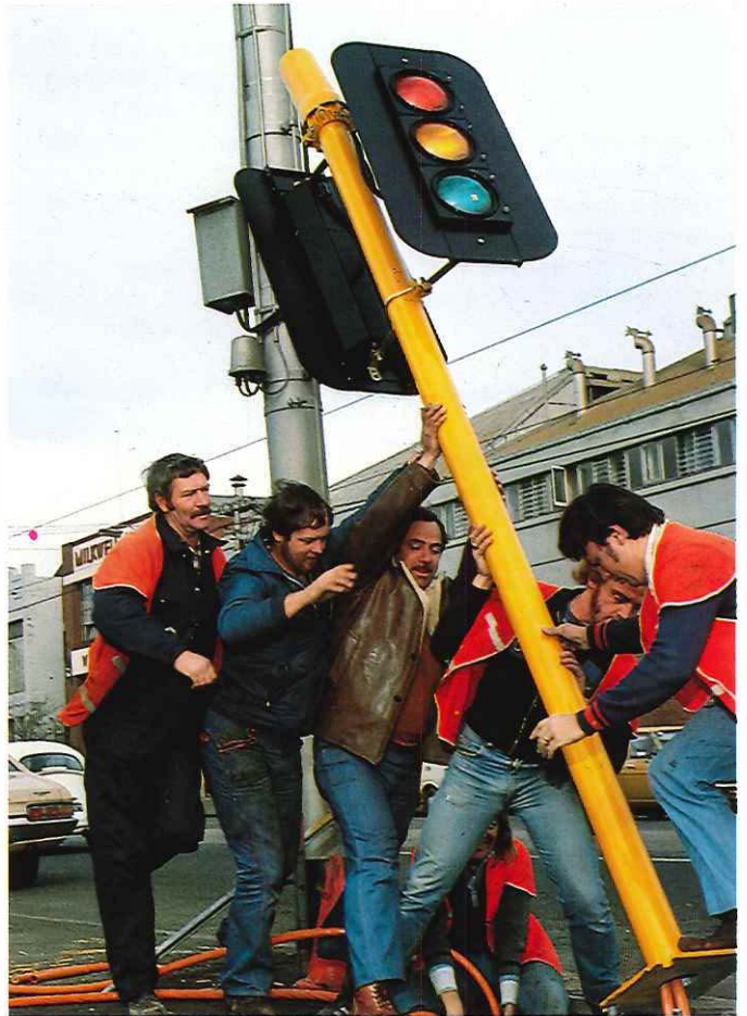
Installation of Advisory Truck Route traffic signals at corner of Clarendon and Grant Streets, South Melbourne.
