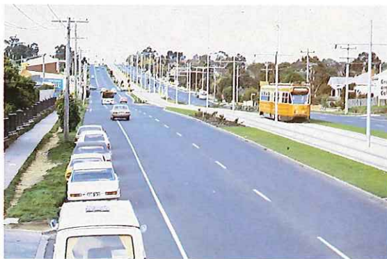
Burwood Highway — completed alterations to highway to allow for extension of tramline from Warrigal Road to Middleborough Road.
