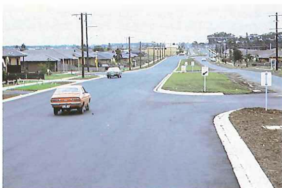
Kings Road, City of Keilor, reconstruction between Gillespie and Taylors Roads (Unclassified Road).
