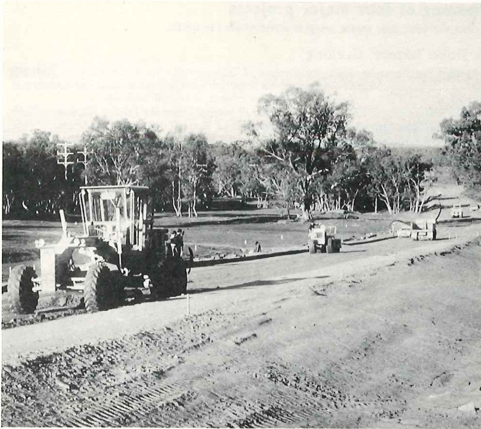
Duplication of the Calder Highway, from Ravenswood to Big Hill, south of Bendigo
