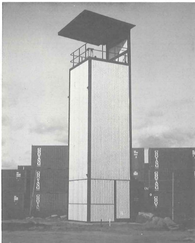
Figure 22 Control survey tower at the elevated section of the West Gate Freeway in South Melbourne
