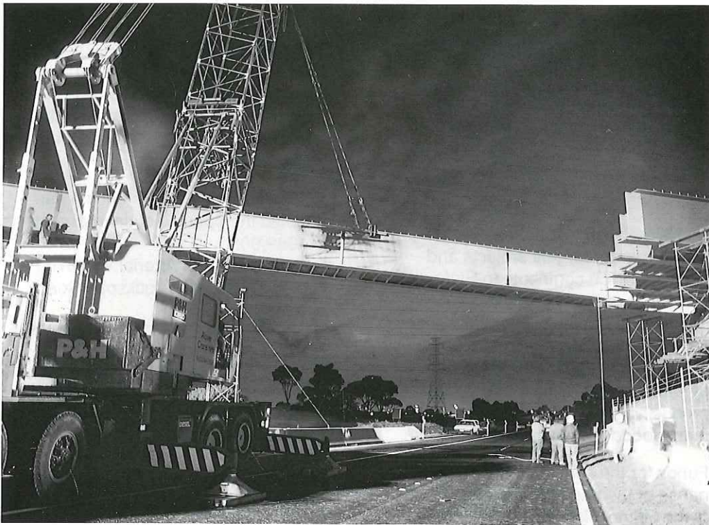
Lifting beams for the Western Ring Road bridge over the Tullamarine Freeway.
