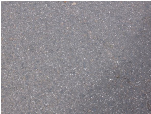
Cracking: slow lane, OWP chainage 143 m
