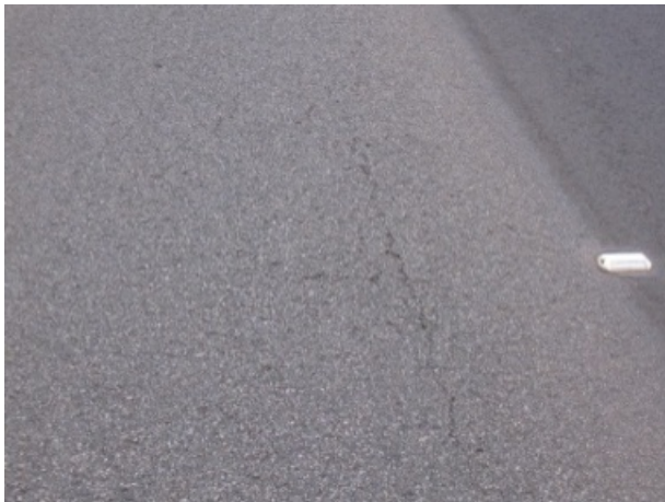
Cracking: slow lane, OWP chainage 611 m
