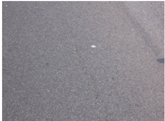
Cracking: slow lane, OWP chainage 292 m
