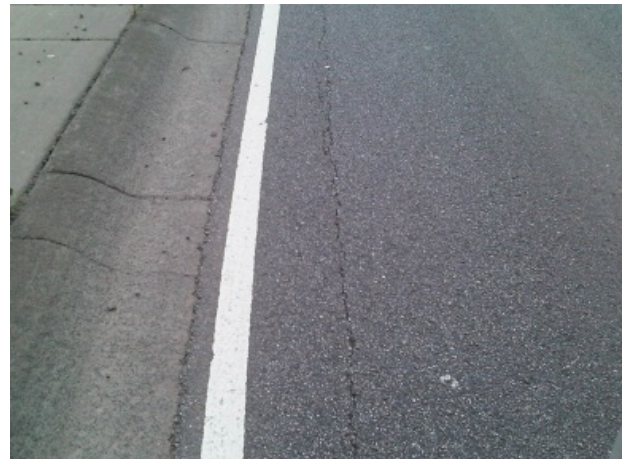
Cracking in fast lane between OWP and kerb
