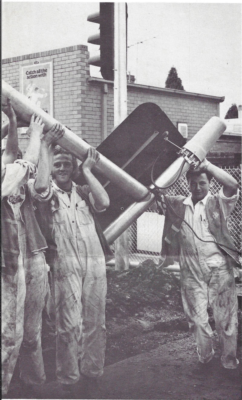
pedestrian lights at Eastern Highway. CRB workmen, from left, Ron Winn, members and Hank Terhorst help to erect the mast as it is o position.
