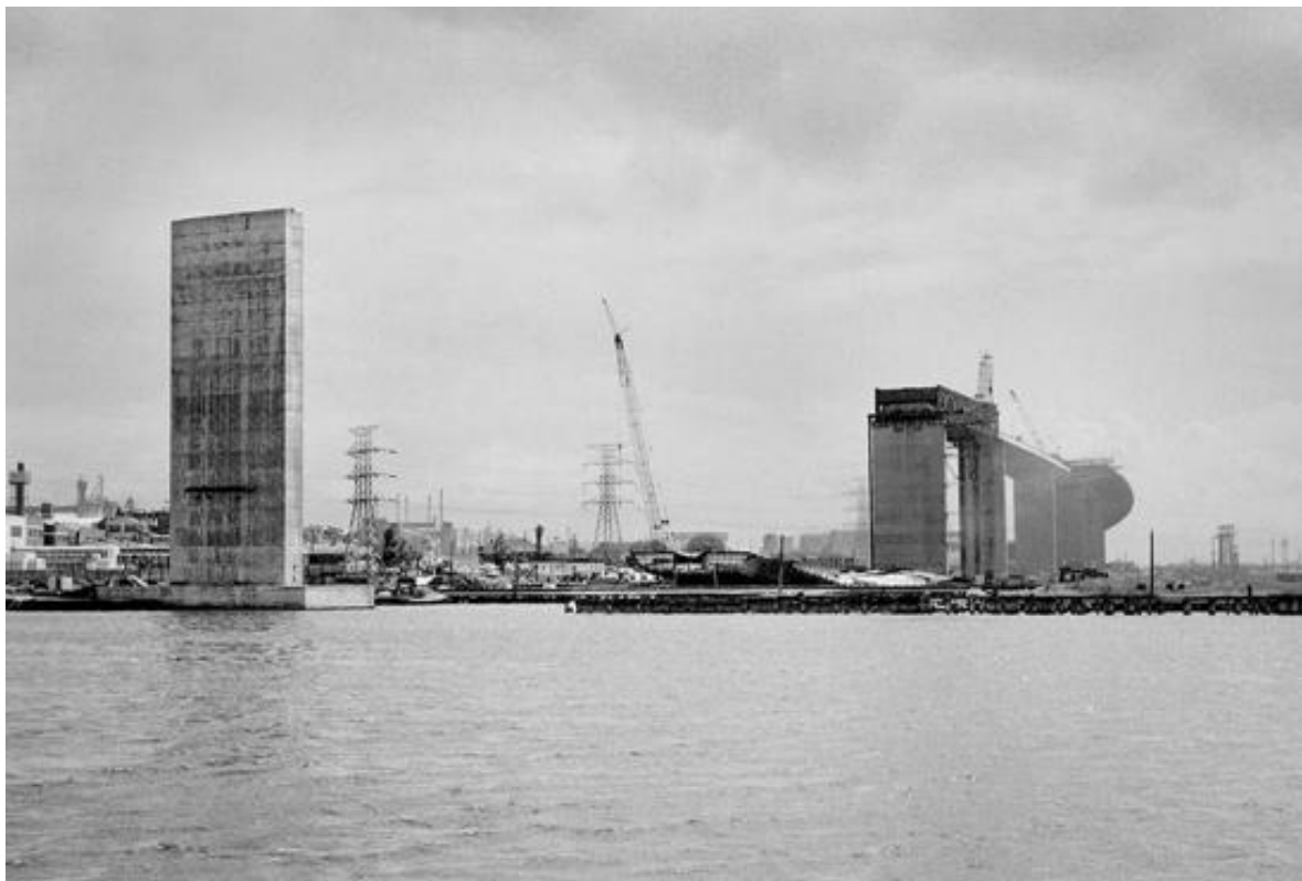
View from the eastern viewing point. Span 10-11 has collapsed, knocking over Pier 11. (Image courtesy of Rob Morgan ARPS)
