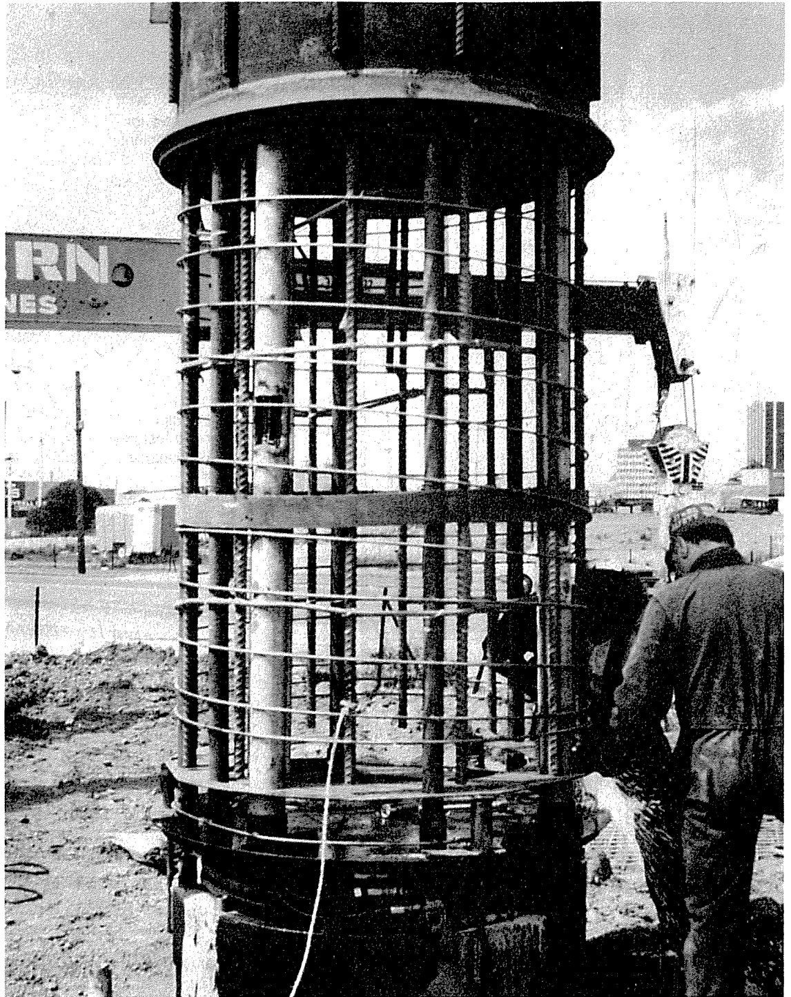
Fig. 7. Strain gauged reinforcement cage and flat jack assembly being lowered into basalt socket
