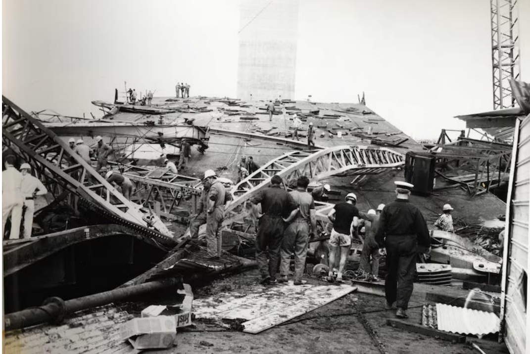
The 2,000-tonne section of the bridge that collapsed in 1970. (Image courtesy of the Public Records Office).
