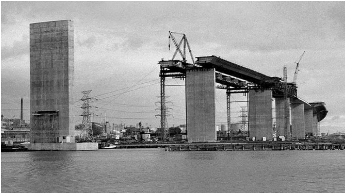
View from the eastern viewing point. Span 10-11 which collapsed in October can be seen in its two halves: the north half up on the piers and the south half jacked up to near full height, ready to be rolled across. (Image courtesy of Rob Morgan ARPS)
