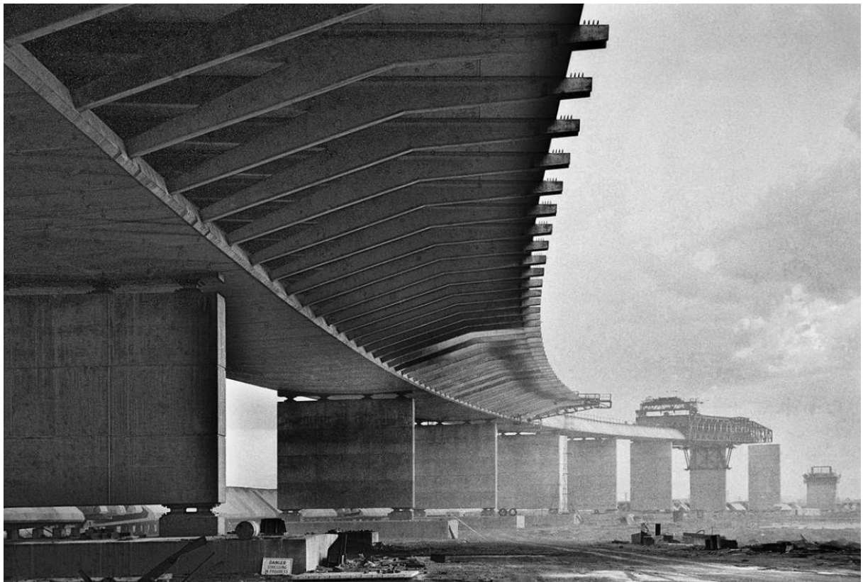
The eastern concrete approach spans being built, viewed from near Todd Road – May 1970. (Image courtesy of Rob Morgan ARPS)
